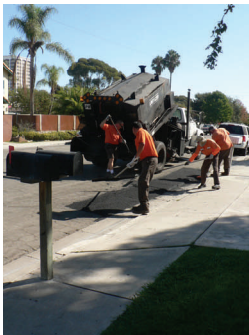
PHOTO: CITY OF COSTA MESA REPAIRS GAPING HOLES AS A CITY IMPROVEMENT PROJECT FOR CENTER
